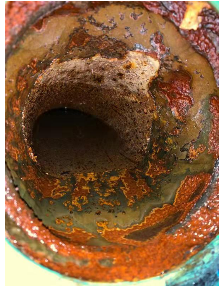
Overboard discharge pipe after 3 month of operation
